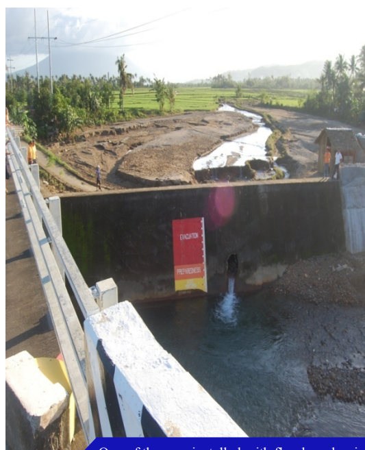
One of the area installed with flood marker in Tiwi. Photo Credits to APSEMO
